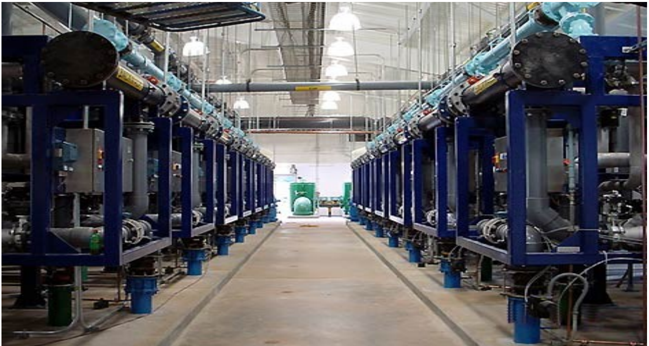
Microfiltration Facility At Ontario
